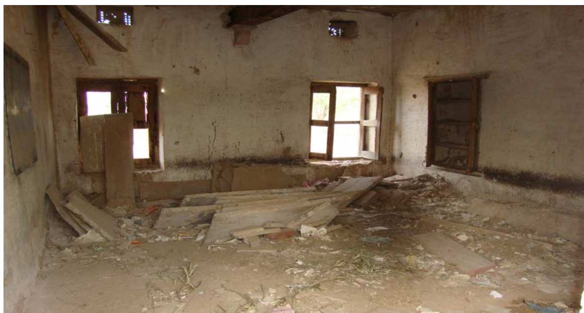
Condition of a room in a school in Churu District
